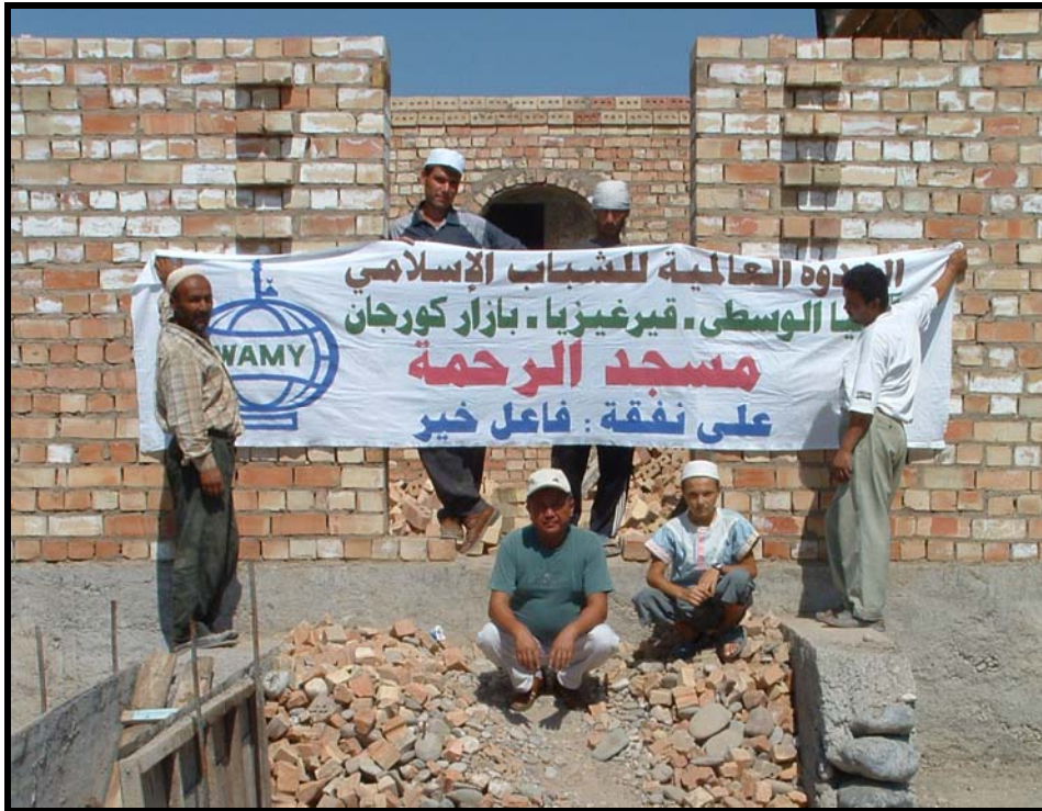
The construction of the 28 th mosque. The banner notes that WAMY and an anonymous donor have sponsored the project.
