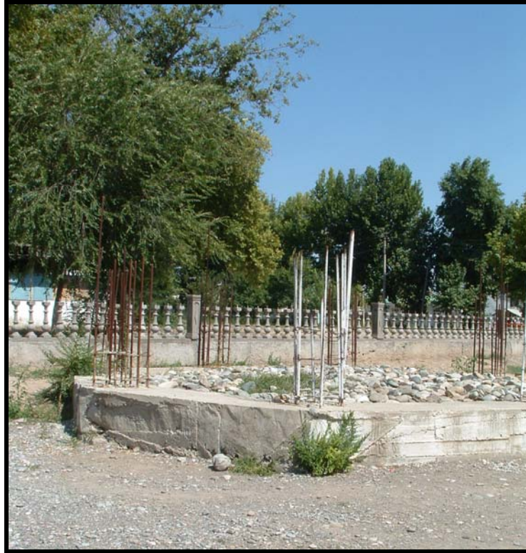
The foundation for the minaret at the Raion Friday Mosque was laid, but never complete. Funds are being sought for the project.
