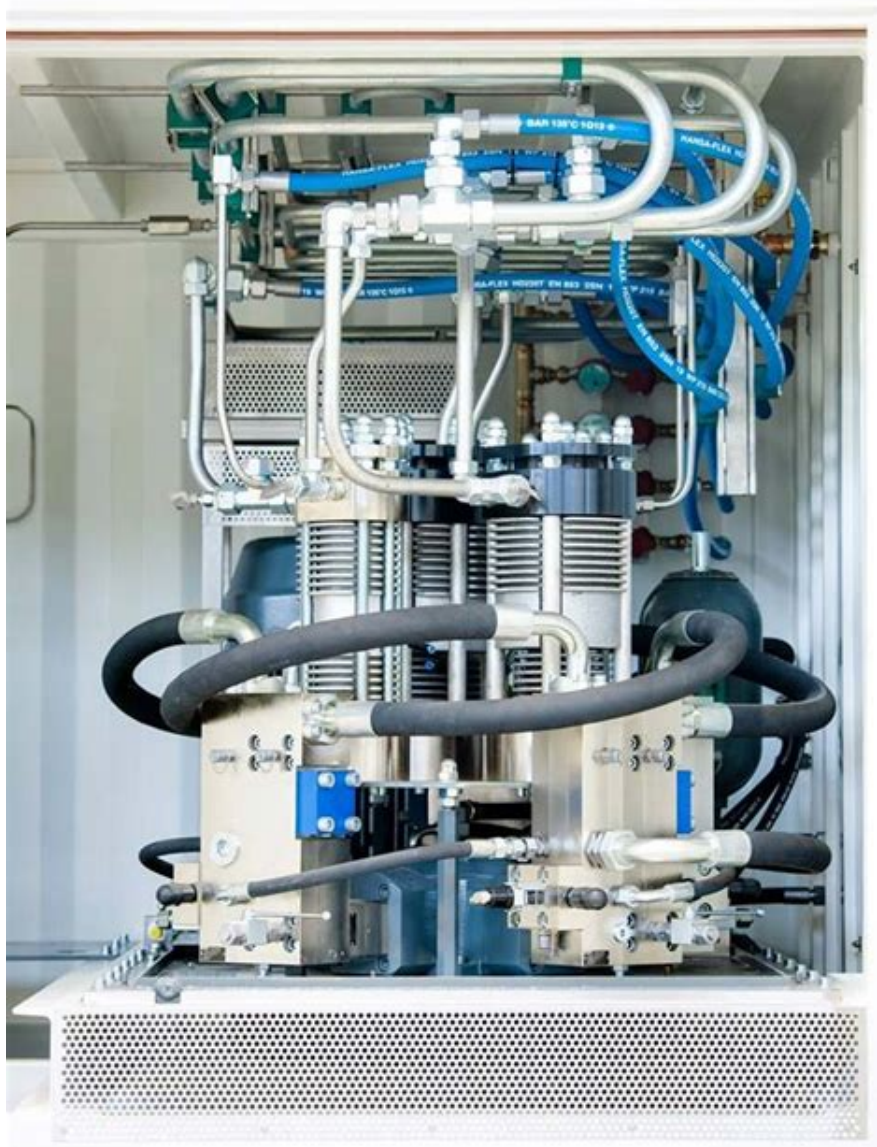
Figure 1.1: Hydrogen compressor unit as part of a hydrogen fuel station engineered by Linde GmbH and run by H2 Mobility Deutschland GmbH & Co. KG [5]. Hydrogen is compressed up to 860 bar and pumped to the dispenser. All the piping is manufactured from austenitic stainless steel AISI 316.
