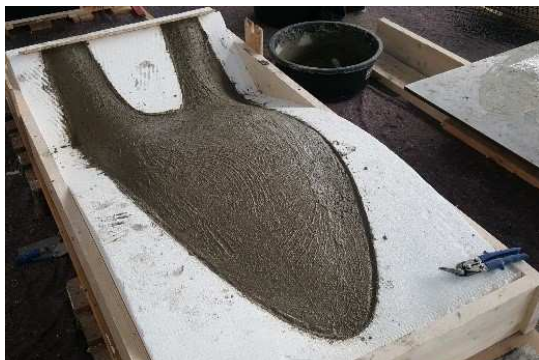
Fig. 32: Laminated concrete surface
