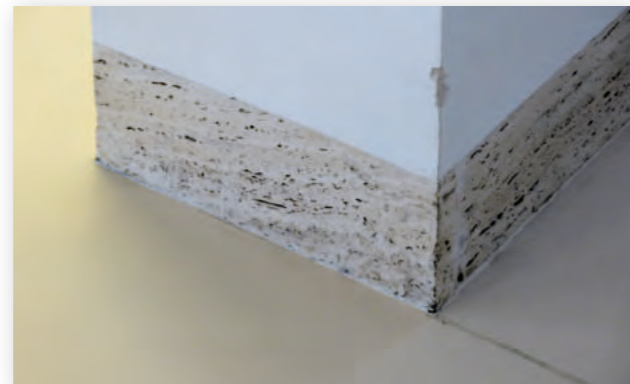
Travertine flush-walled skirting boards
