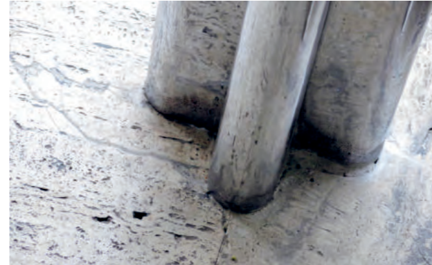
The point where the cross-shaped steel supports meet the travertine floor covering
