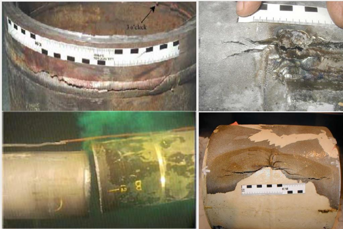
Figure 2-20: Failures in the TUNE pipeline that occurred due to HAC. The right side photos present failure of the weld due to hydrogen absorbed during welding process. The left side photos present failure induced after the reparation and coating process. Hydrogen was introduced through gaps in the coating and the cathodic protection that was applied to the flowline [23]
