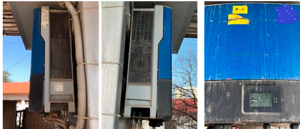
Figure 4. Example of inverter malfunction due to soiling accumulation leading to fan failure and hence overheating.
