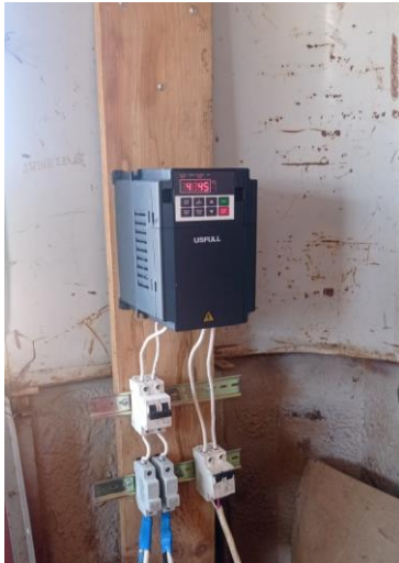
Figure 5: Overview of lightning-protected PES and electronic devices.
