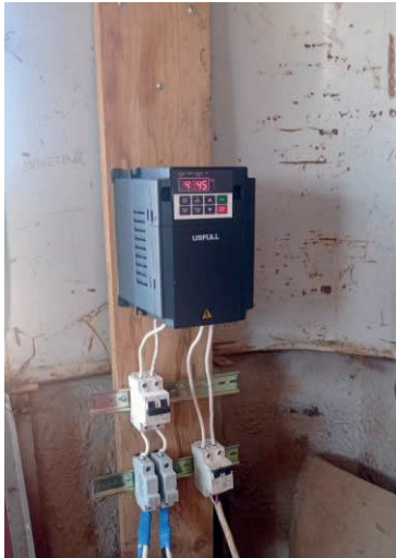
Figure 5: Overview of lightning-protected PES and electronic devices.
