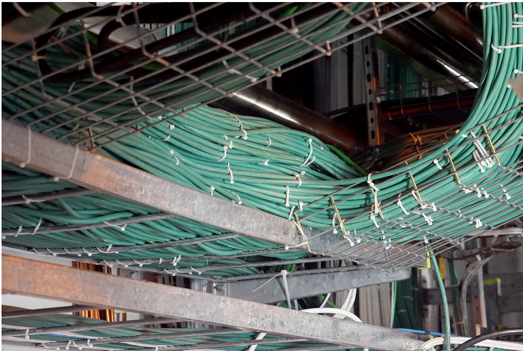
Figure 2.4: Example cable tray in UXC55 (Picture taken in February 2015).
