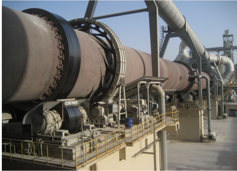
Fig.1 Rotary Kiln ( \Phi 6.2 \times 98\text{m} ) of a Clinker Production Line (Ch1)
