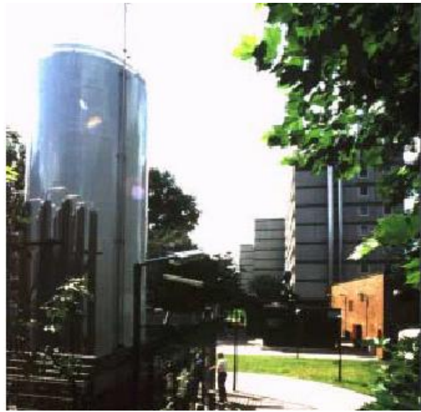
Figure 3.14 The FC-CHP plant at Lysierstrasse in Hamburg-Bahrenfeld [166]
