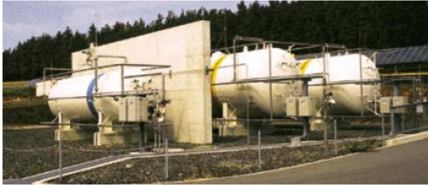
Figure 3.4 GH2 storage at the solar-hydrogen plant [215].
