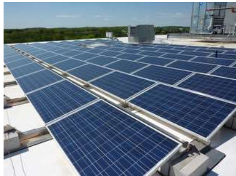
Solar Panel Water Heater
