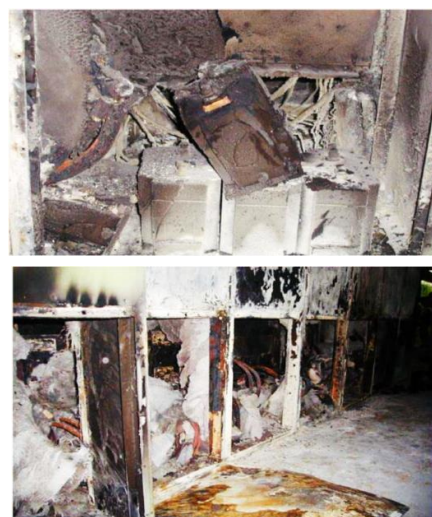
Figure 1: Damage to the voltage transformer.
